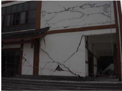
Figure 1: Shear damages observed in load bearing walls of unreinforced masonry buildings and masonry infill of concrete buildings due to earthquake induced lateral loads.
