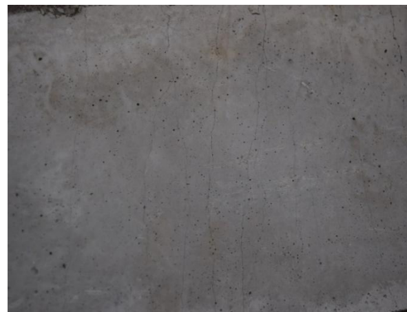
Figure 11: Picture shows micro cracks generated in ECC
