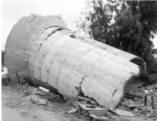
Figure-2: Collapse of water tank in Bhuj
